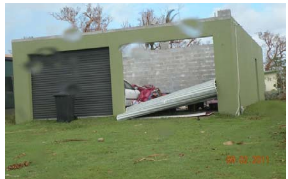
A roller door failure leading to roof failure
