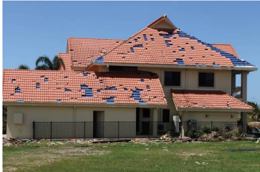
Extensive tile damage on a modern house
