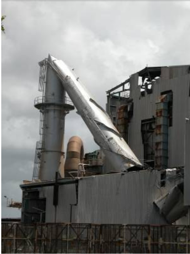
Collapsed chimney stack - Mourilyan Sugar Mill, (image courtesy of John Holmes)
