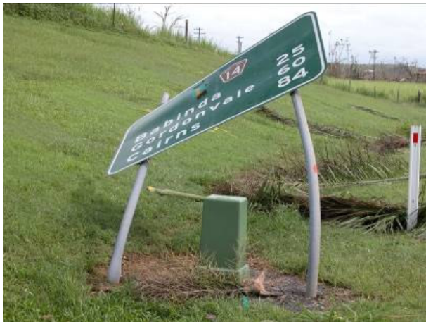
Failed Road Sign – used to determine Gust wind speeds (image courtesy of John Holmes)
