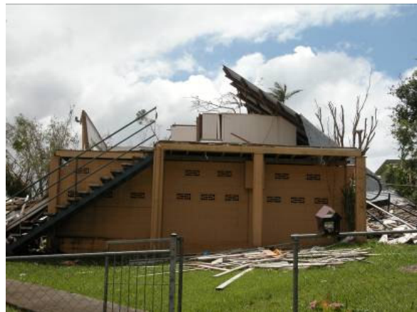
Near complete destruction of high-set house, East Innisfail (image courtesy of John Holmes)
