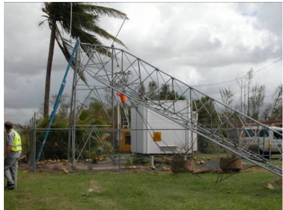
Failed Communications Tower, Silkwood (image courtesy of John Holmes)
