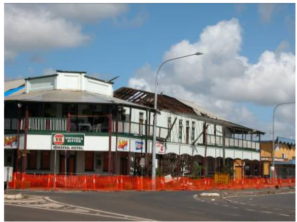
Innisfail Hotel, with extensive roof damage (image courtesy of John Holmes)
