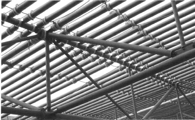
Figure 1: Array of CHS members showing failures and temporary restraining ropes
