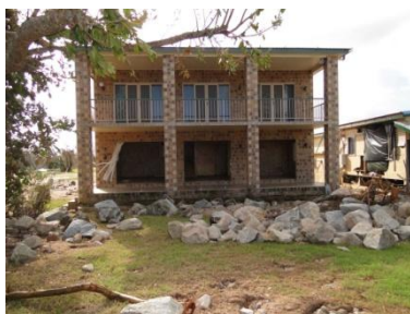
Figure 7. 2 Storey house on seaward side of road at Tully Heads. (Same property as Figure 6)
