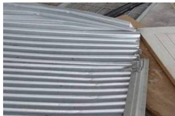
Figure 4: Roller door guide failure
