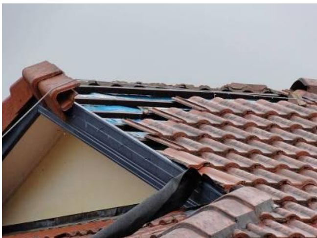
Figure 6: Failure of ridge capping
