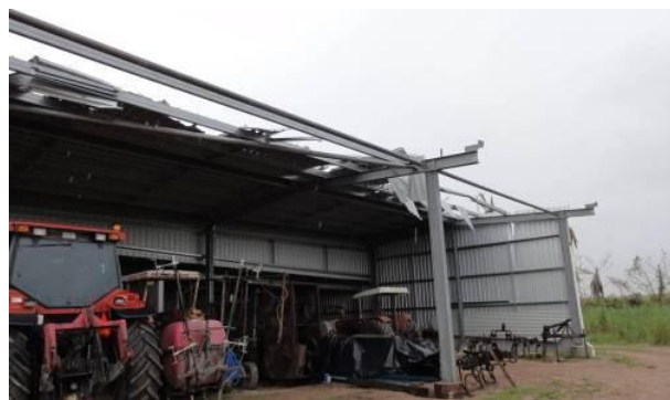
Figure 7: Buckling and loss of purlins with cladding
