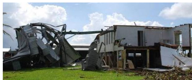
Figure 8: Failure of shed and impacted house
