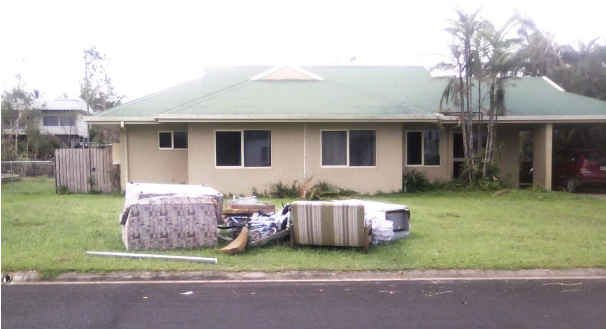
Figure 7. A house with little exterior damage. The pile of water damaged contents and linings on the nature strip is indicative of significant water ingress damage that would not be detected if the materials and goods had been removed.
