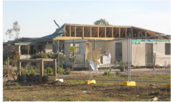
Figure 5. Roof damage – Sun Country Holiday Village, Mulwala
