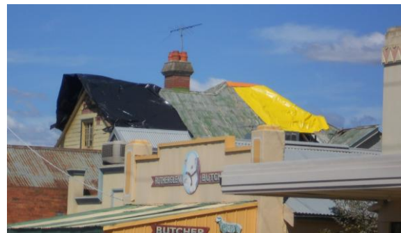
Figure 11. Roof damage – Rutherglen, Victoria
