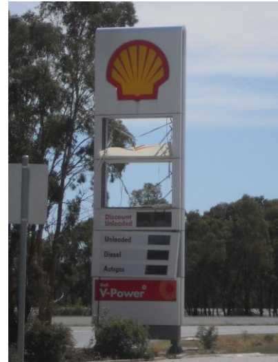
Figure 13. Panel damage – Shell service station, Euroa, Victoria
