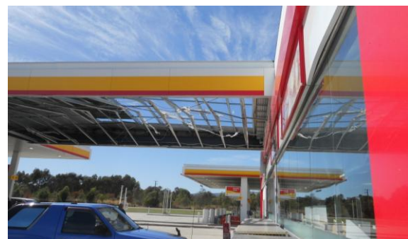
Figure 12. Soffit and canopy damage – Shell service station, Euroa, Victoria
