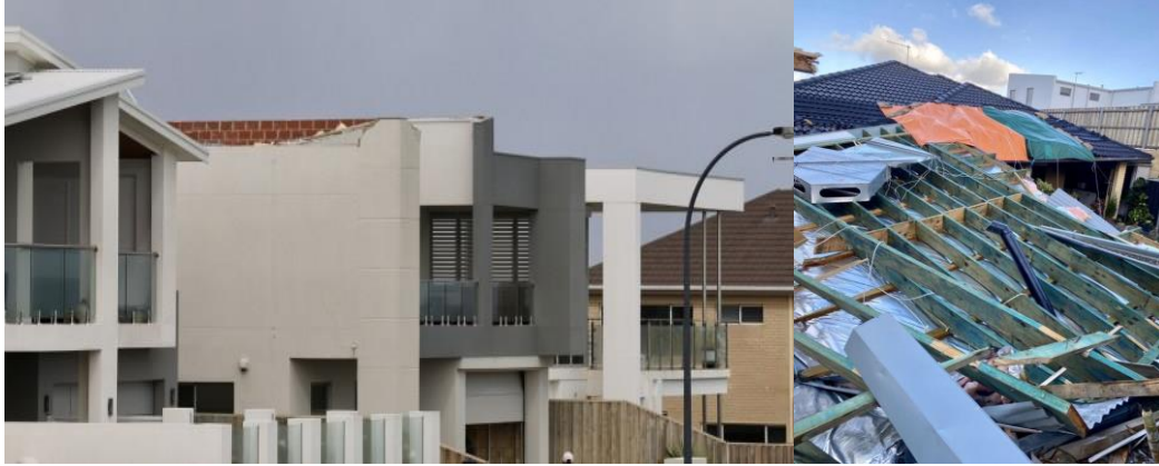
Figure 3: Wind damage to skillion roof buildings
