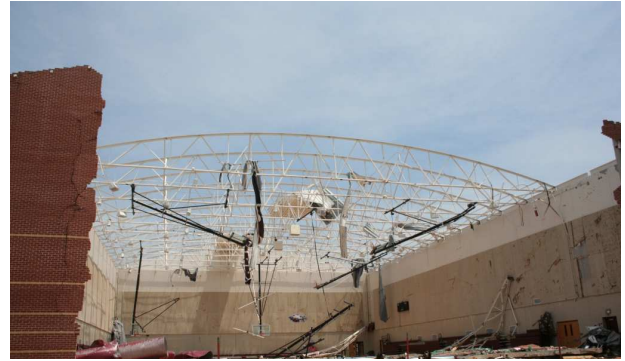
Figure 3 Damaged school in Joplin, MO USA
