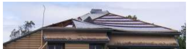
Figure 2. Roof cladding section flipped to leeward side with battens still attached.
