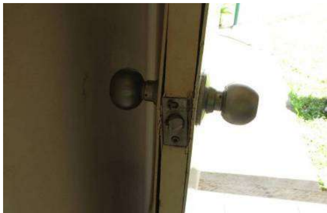
Figure 3. Typical lock and damaged door after being blown inward during Cyclone Yasi in 2011.
