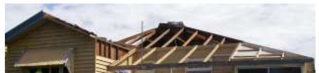
Figure 1. Removal of roof cladding and battens from the windward face of a residential structure.
