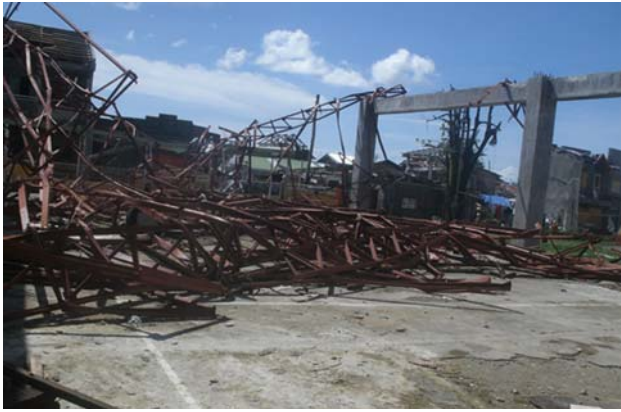
Figure 3. Collapsed Steel roof of a multi-purpose covered court (photo from ICE-PICE-JSCE Joint Survey).
