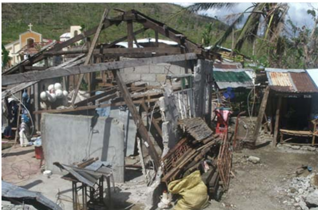
Figure 4. Typical damage to a one-storey CHB residential house with wooden truss (photo from ICE-PICE-JSCE Joint Survey).
