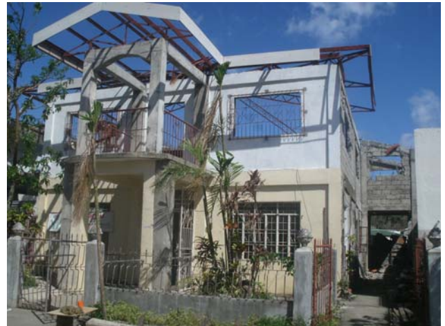
Figure 1. Typical damage to a two-storey reinforced concrete building (photo from ICE-PICE-JSCE Joint Survey).
