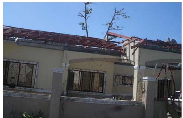
Figure 2. Typical damage to a one-storey reinforced concrete residential house (photo from ICE-PICE-JSCE Joint Survey).
