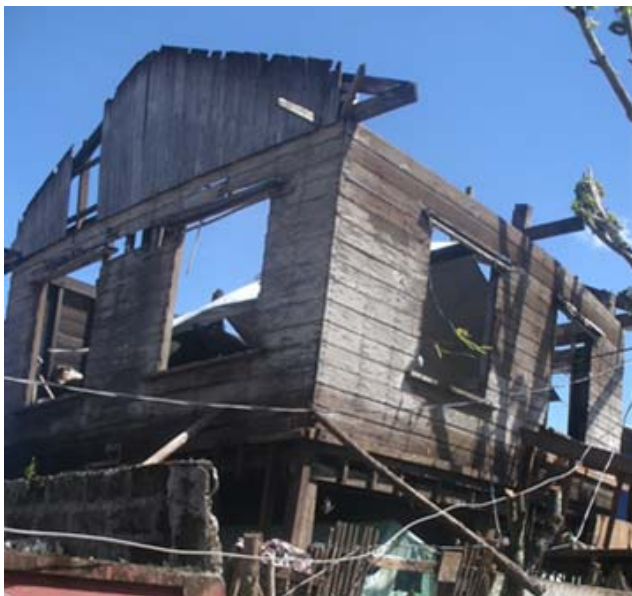
Figure 5. Typical damage to a two-storey wooden residential house (photo from ICE-PICE-JSCE Joint Survey).
