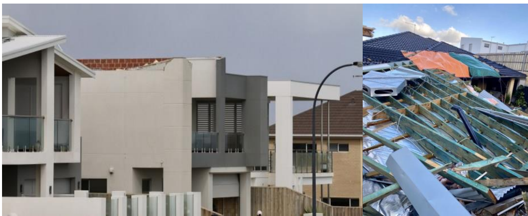
Figure 3: Wind damage to skillion roof buildings
