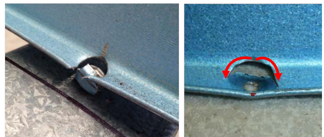
Figure 2. Pull-through Failures of Roof Battens
