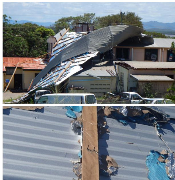
Figure 6. Loss of roof from older property. Cladding had been replaced but no retrofits or upgrading of batten to rafter connections observed.
