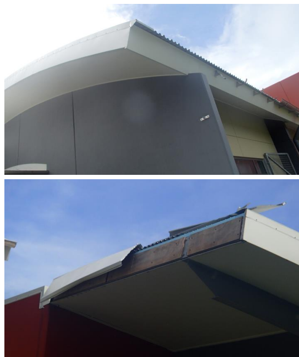
Figure 7. Failed (a) gutter and (b) flashings on modern community shelter
