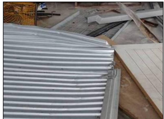
Figure 2. Failure of a garage door with wind locks installed and still engaged in the guides, but has become detached from the support structure (Boughton et al., 2011).
