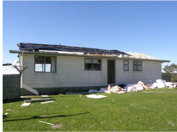
Figure 5. Roof damaged in Northland storm
