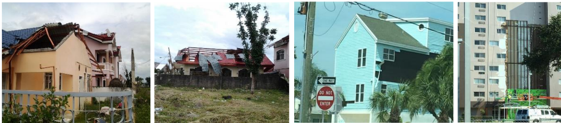
Figure 1. Typical damage from cyclones and hurricanes to non-structural elements. Left – damage to tiled roof section including sheathing, typhoon Haiyan, Tacloban; Second Left – extensive damage to metal roofing panels, typhoon Haiyan, Tacloban; Third Left – wall cladding damage, hurricane Irma, Florida; Right – collapsed EIFS cladding panels, hurricane Irma, Florida. (RMS Photos)
