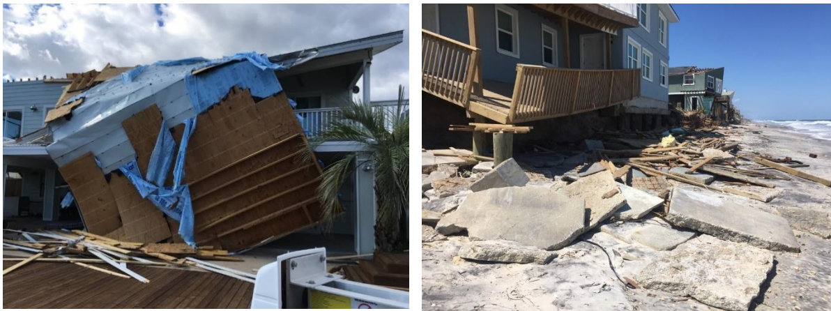
Figure 3. Roofing failure due to failed roof/wall connection in Hurricane Harvey (left) and severe storm surge damage along Northeast coast of Florida from Hurricane Irma (right)
