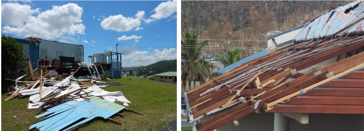
Figure 4. Roofing failure due to failed roof/wall connection in Cyclone Marcia (left) and failure at batten/rafter connection from Cyclone Debbie (right)
