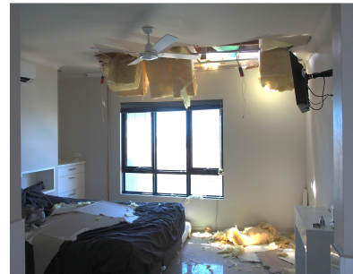
Figure 1. Water damage to linings
