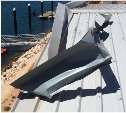
Figure 3. Loss of barge flashing
