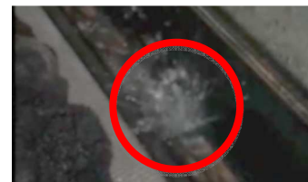
Figure 2. Water penetration through weep hole in window (photo by home owner)
