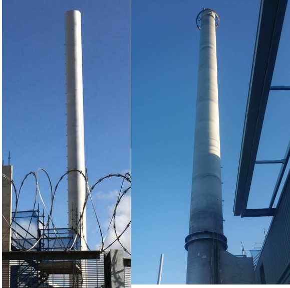
Figure 1: Photo of stack before (L) and after installation of damper (R)
