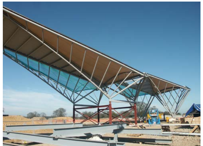
Fig 6 Ascot Racecourse redevelopment, roof trial assembly showing fabric hypar and metal clad sections.
