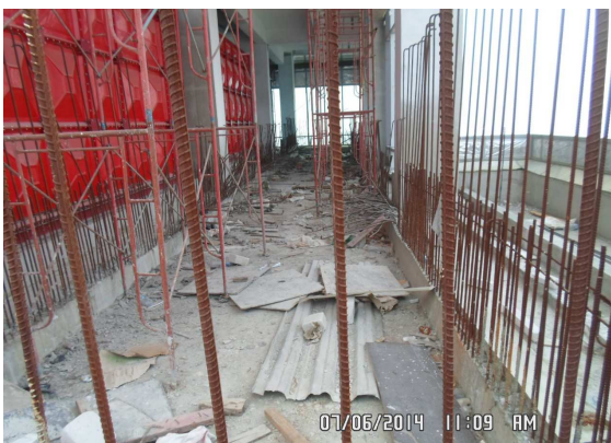
Figure 3. One of 2 allocated spaces for the Hybrid TLCD/TLSD system.
