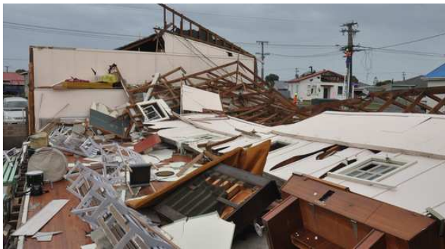
Figure 5. Greymouth Band Hall in Blaketown destroyed.
