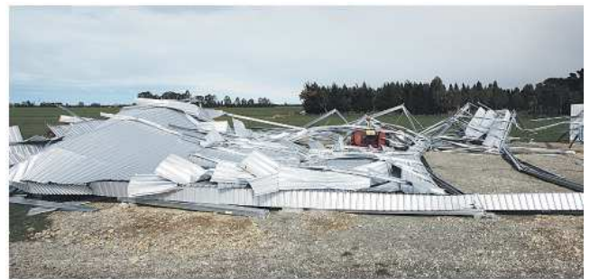
Figure 3. Agricultural building destroyed.
