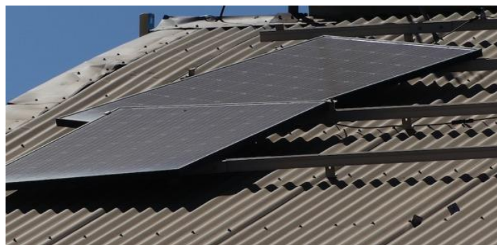
Figure 3. Failure of clips on roof-mounted PV arrays
