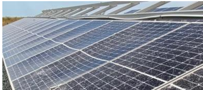
Figure 2. Examples of failure of ground-mounted solar panels
