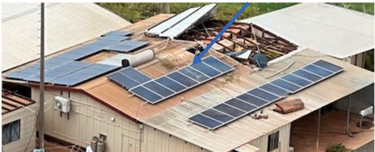
Figure 5. Damage to batten fixings under roof-mounted solar panels in TC Ilsa WA 2023
