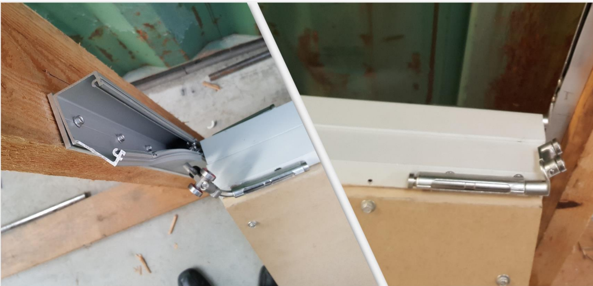
Figure 3. Bi-fold hardware failure well below serviceability loads.
