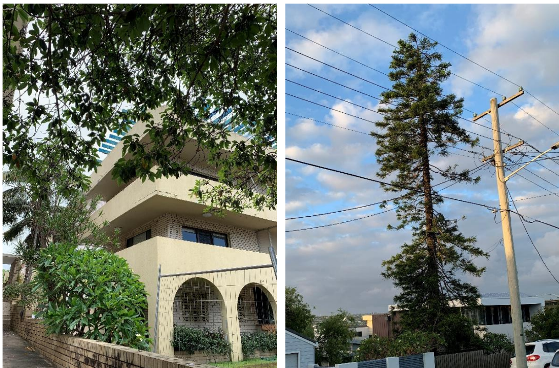
Figure 5: Unit block on Pacific Pde lost its roof yet suffered no damage at ground level (L). Branches snapped from the central 1/3 of a Norfolk Island Pine (R).
