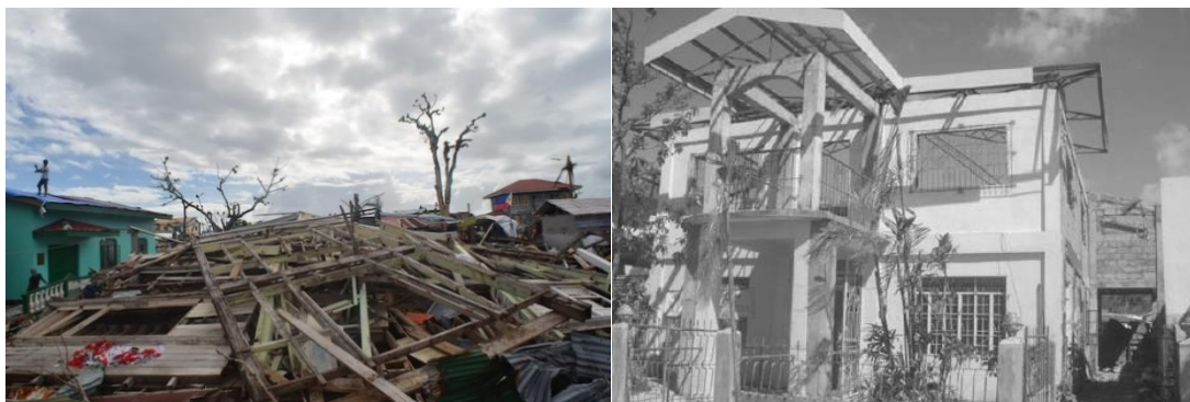
Figure 1. Extensive Damage on Light Frame Wood Structures vs Roof Damage on Concrete Structures
